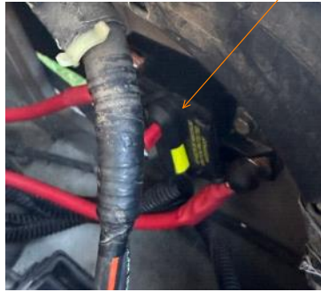
Step 2) Blue Sea 60 amp breaker in engine compartment Battery line runs to here. From here into RV
