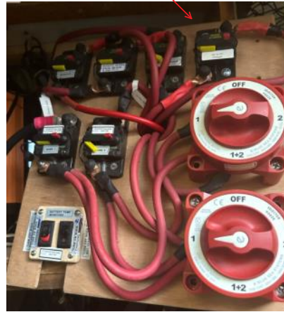
Broader view of system (Two lithium banks, each 200 amp hours. Smart Shunts etc.) DC to DC breaker in last image
