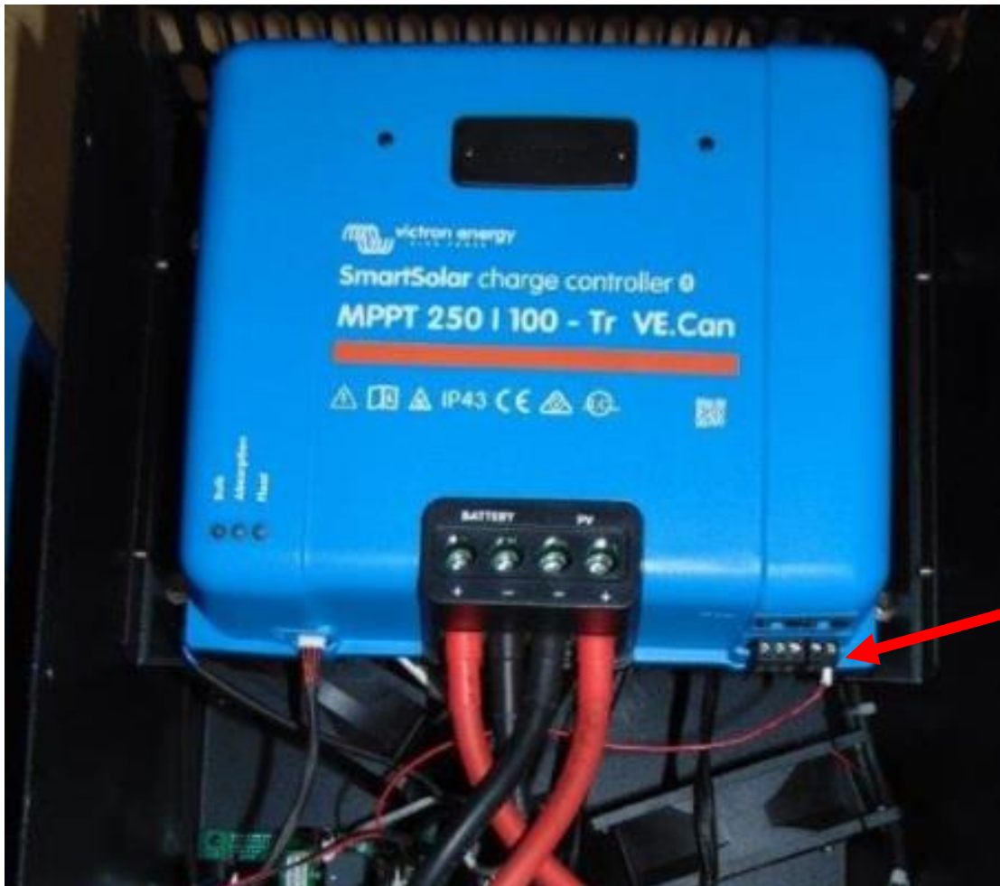
The photo above shows a wrong connection of the thin red wire to the port L instead of H
